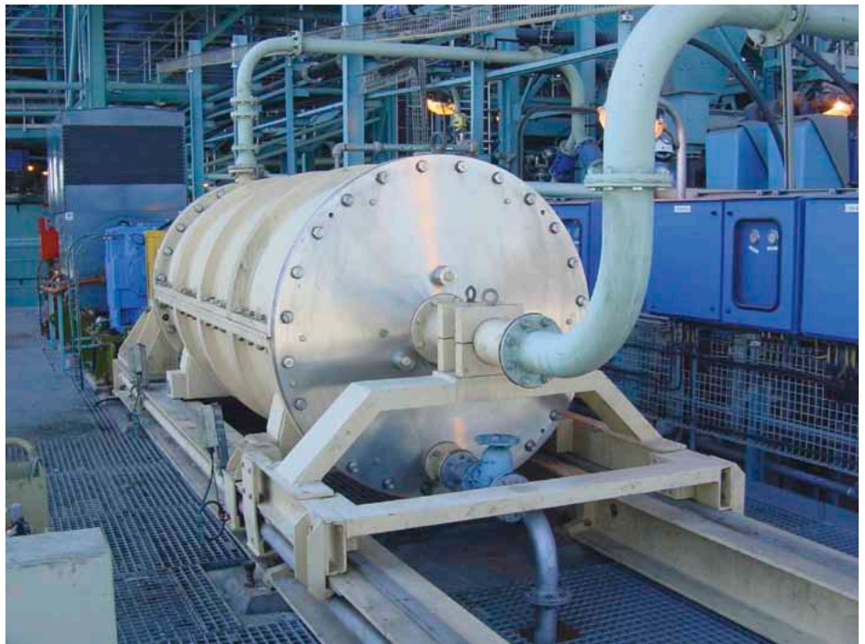
The first Lonmin IsaMill™ (M3000) operating at the EP-C Concentrator
